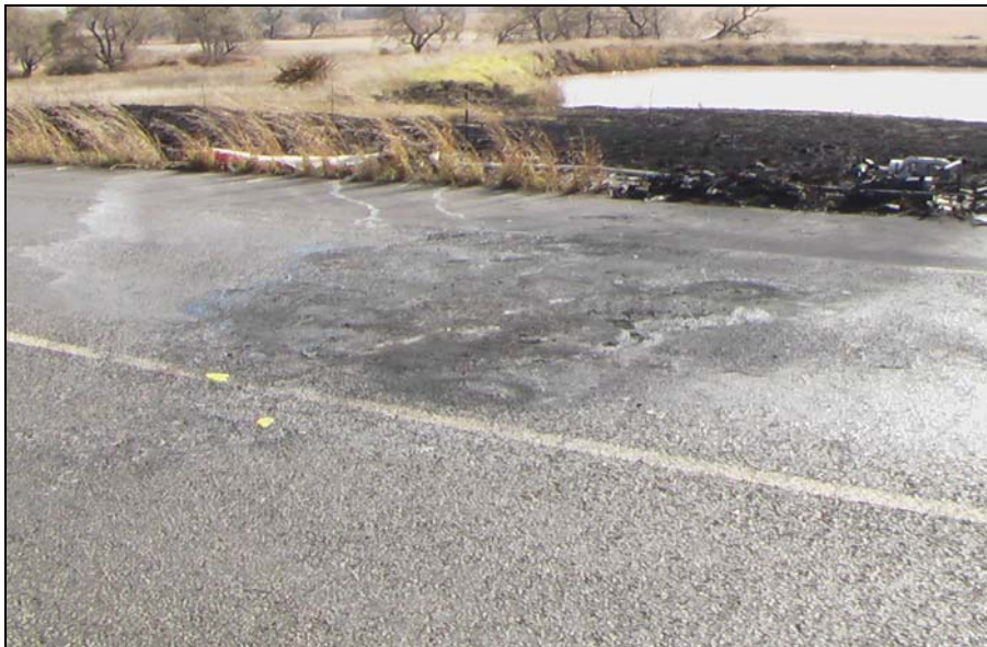
PHOTO5 : VIEW OF DAMAGE TO TAR ROAD BY THE ENSUING FIRE
