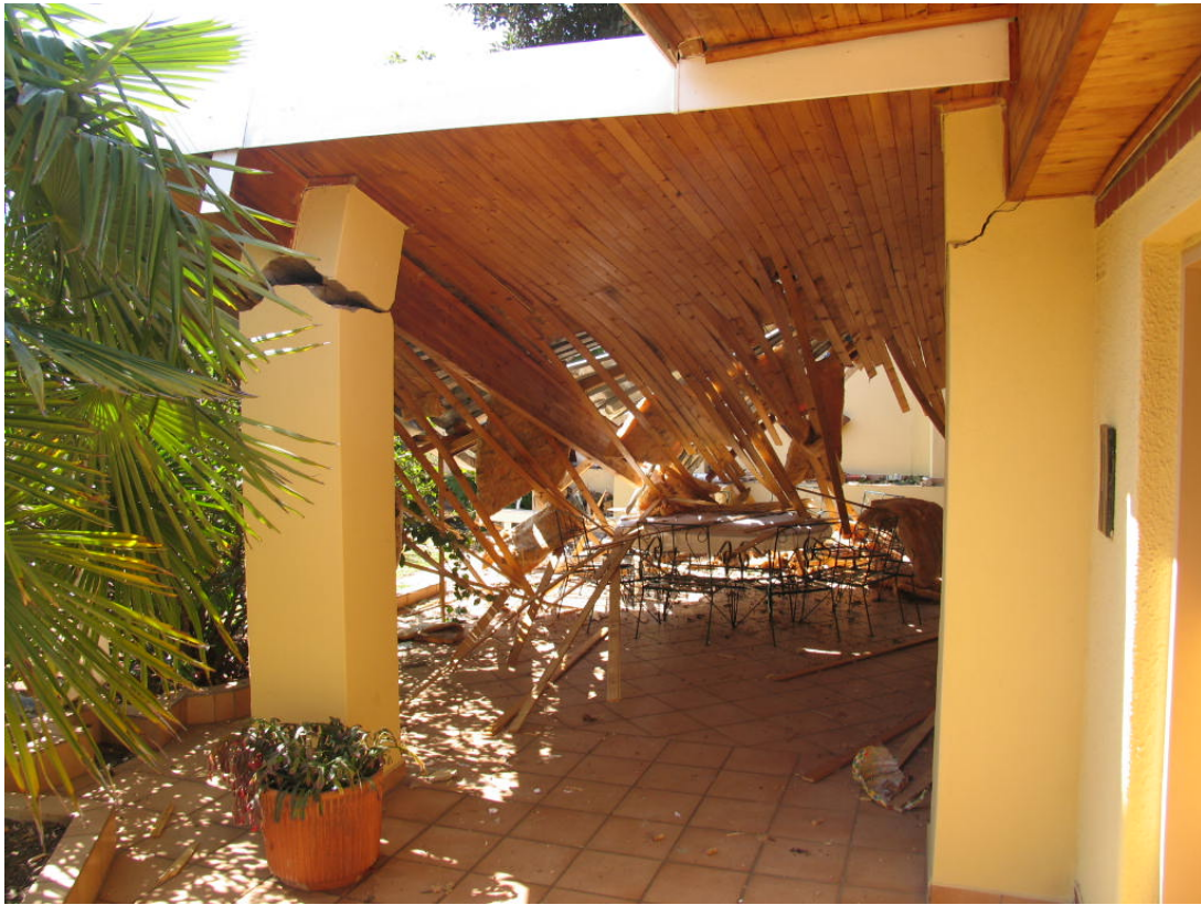
Figure 3. Structural damage to the entertainment area.
