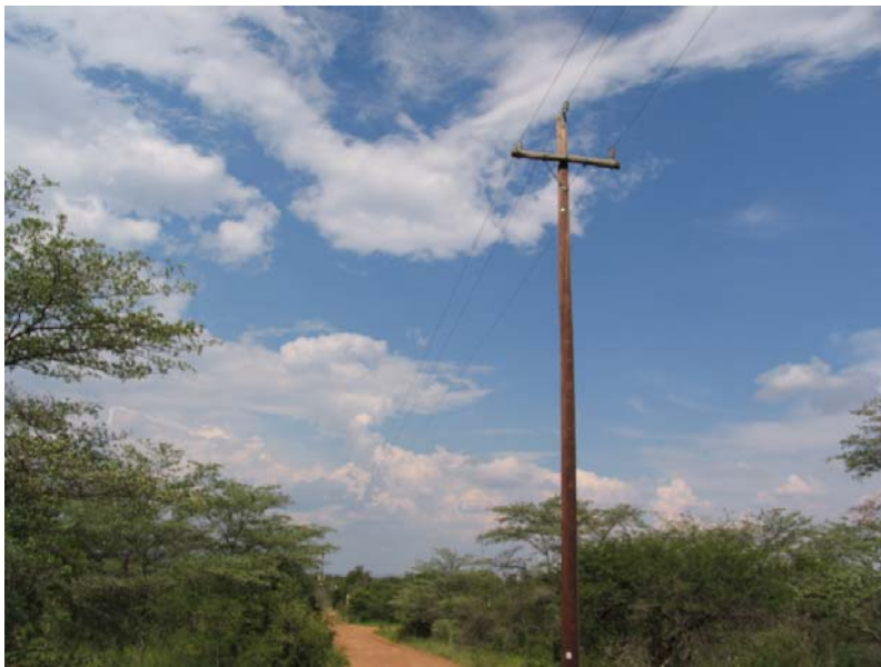
Figure 2. A view of the power lines in question, which were 10m (33 feet) in height.
