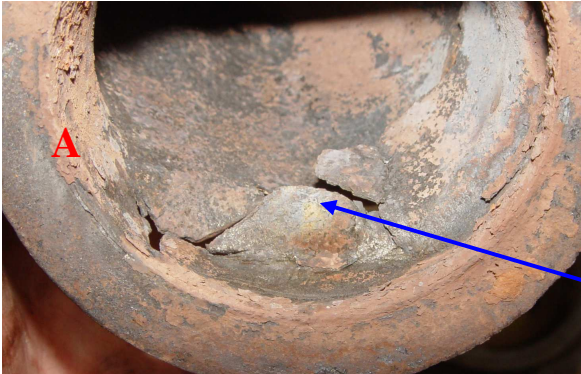
Photo 8: Turbocharger A, exhaust outlet duct, inner area showing fractures (digital)
