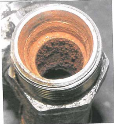
Photo 7: Inner area of t-piece showing corrosion products (digital)
