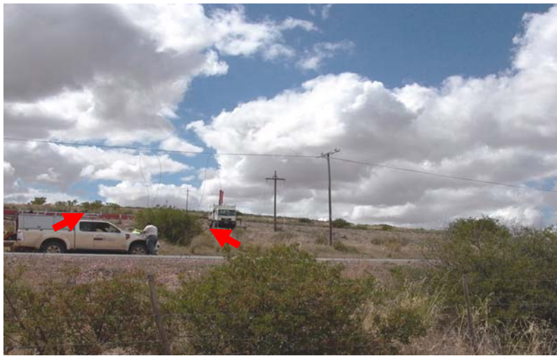
Figure 1. The damaged power lines alongside the road.
