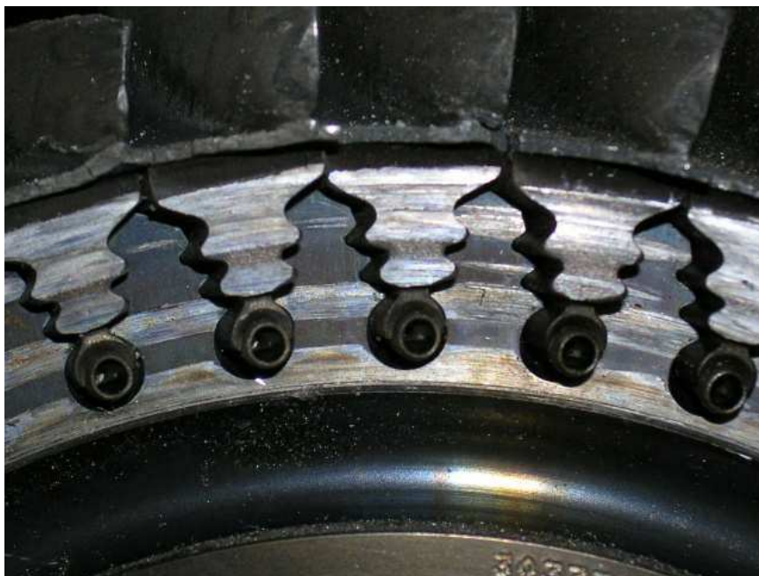
Photo No. 16 2nd stage power turbine downstream side, detail
