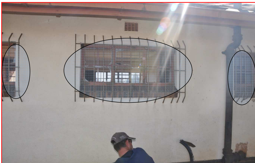
Figure 4: Damage to the Caretakers Office
