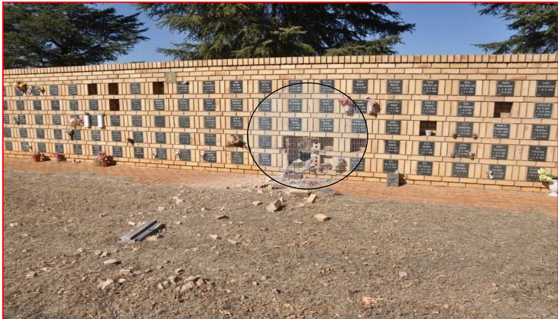
Figure3: Shows damage to the “Wall of Remembrance”
