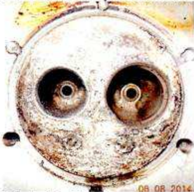
Photo 17: No 2 head damages (digital)
