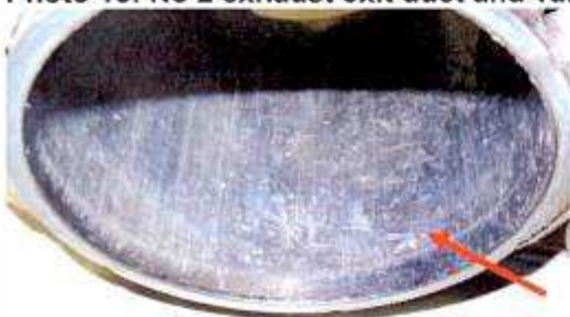
Photo 19: No 2 pod damages (digital)
