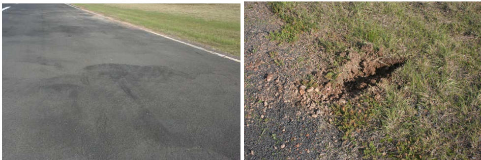
Figure 2 Scratch marks on the runway and the damage caused by propeller strike
