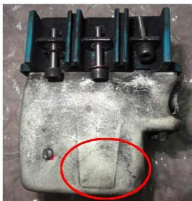
Figure 19. RCCB 991JV6 exterior dried fluid
