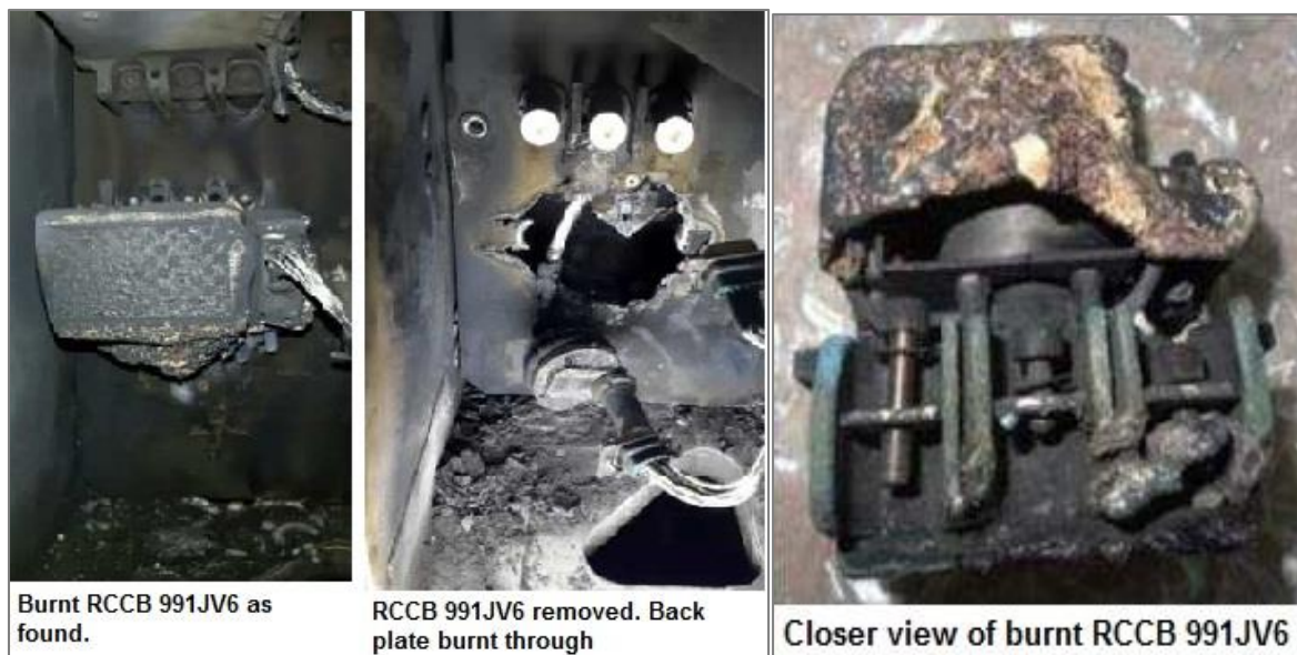
Figure 2. Burnt RCCB 991JV6
