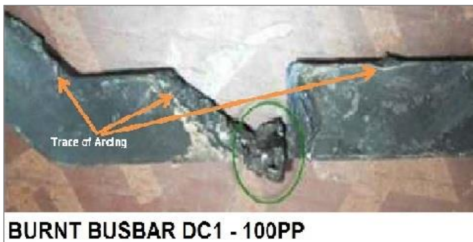
Figure 3. Burnt Busbar 100PP
