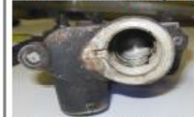
Photo 17: Internal area - Hydraulic Control Valve (digital)
