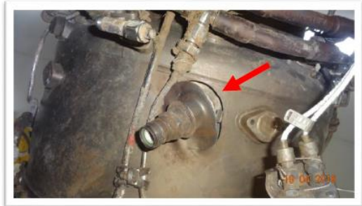
Image #11: Igniter boss appears to have partially parted from Combustion Chamber.
