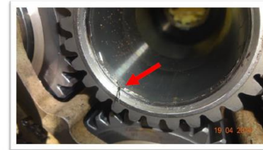
Image #16: Abnormal wear noted on the Sun Gear, possibly caused by rub from the Propeller Shaft.
