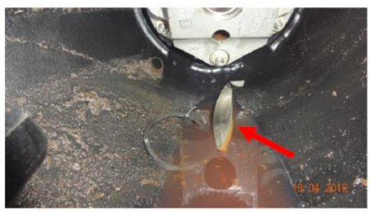
Image #17: Large metal debris found in the Accessory Housing suspected origin from the No. 1 Bearing Assembly.
