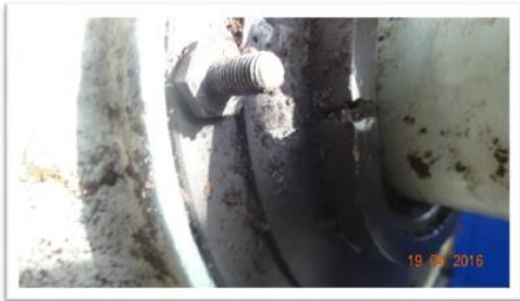
Image #5: Output Housing Carbon Seal Carrier severely damaged.
