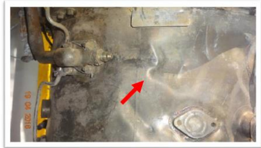
Image #12: Combustion Chamber has been distorted in numerous areas.
