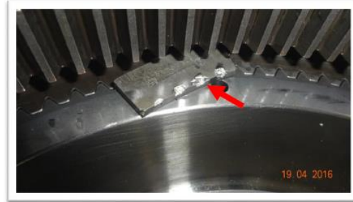
Image #14: Abnormal wear noted on the retention plate retaining the ring gear.
