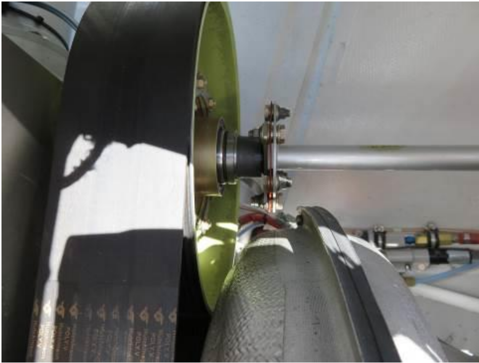
Figure 8. The drive belt and drive train remained intact
