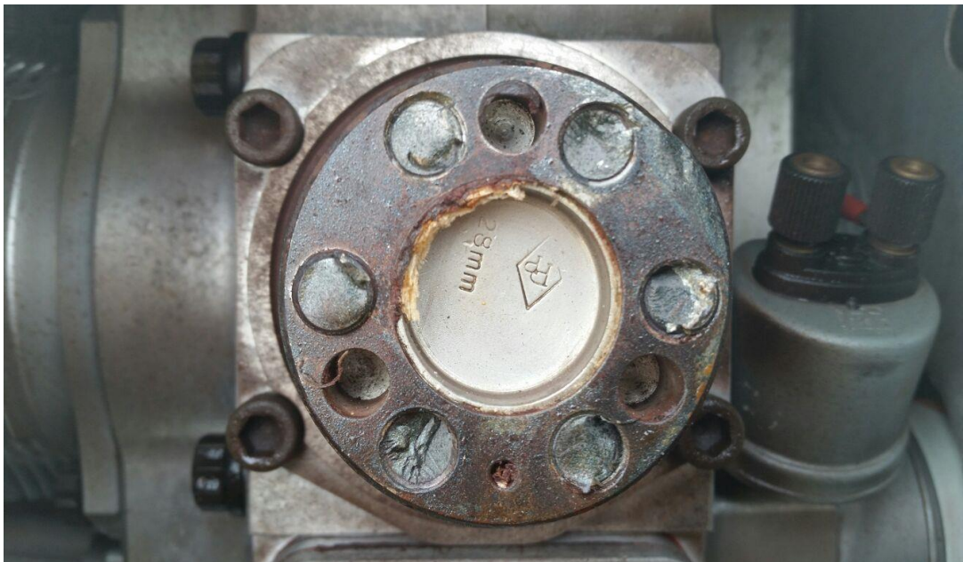
Figure 2: The crankshaft flange with the sheared propeller bolts visible
