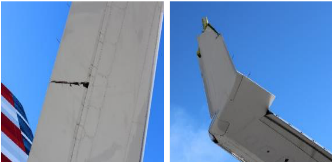
Figure 3. Photograph of the cut in the right elevator of aircraft N758AN (left) and of the left wingtip of aircraft EC-LZX (right)
