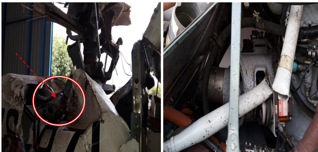
Figure 10: A photograph showing a detached hydraulic actuators and a damaged engine support bar
