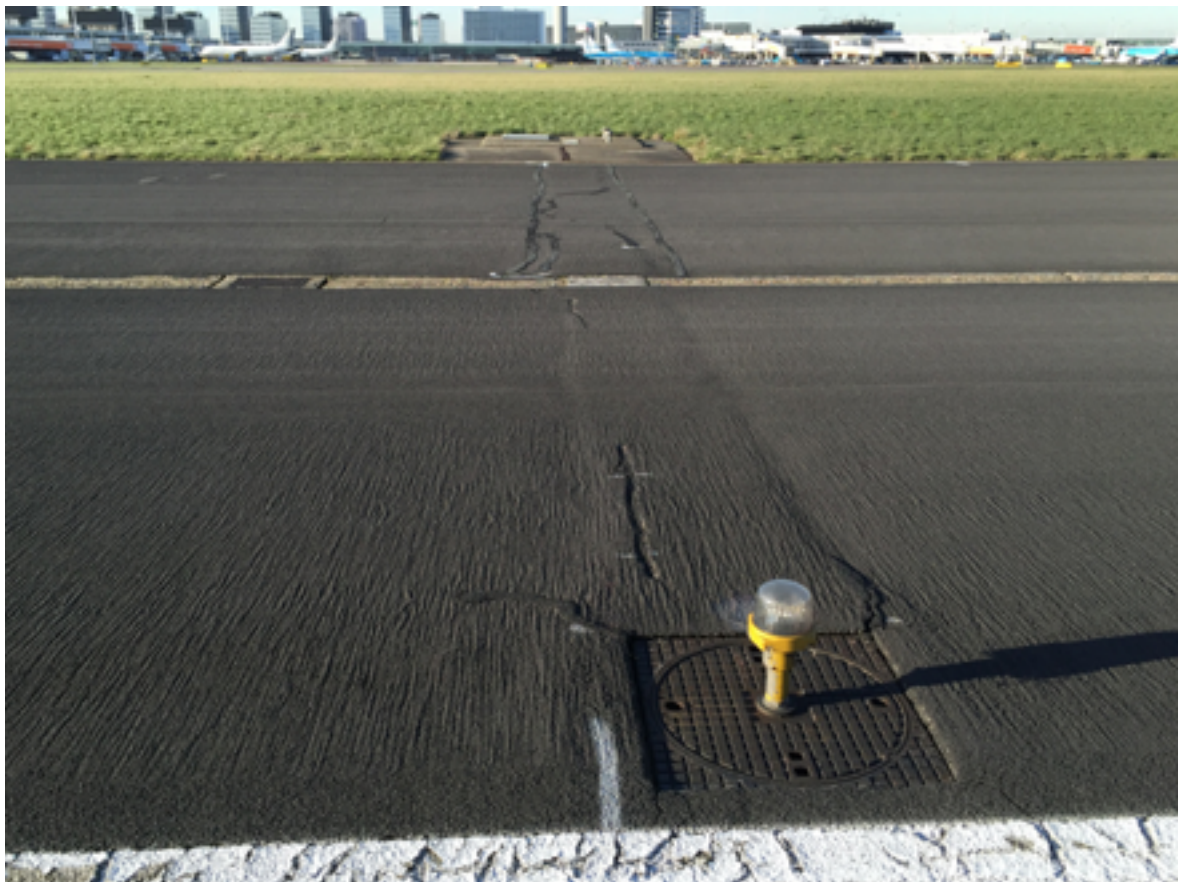
Figure 8: Runway edge light as located alongside Runway 06/24 at Amsterdam Airport Schiphol.
