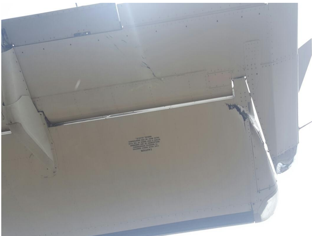
Figure: 4 The damaged aileron of the RH wing of the ATR-72-212A (600 version) aircraft
