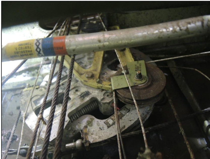
Figure 41 - Overview of the central quadrant on the aircraft floor with oxidation signs on the control cables of the primary surfaces and the compensators.
