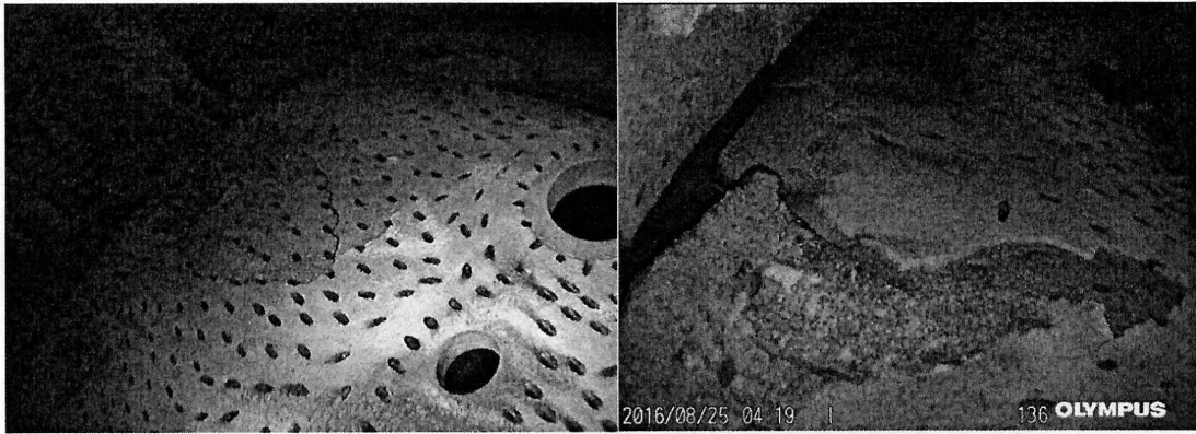
Figure 1 Unchanged 1" Cracks in IBL2 on 24th August 2016
