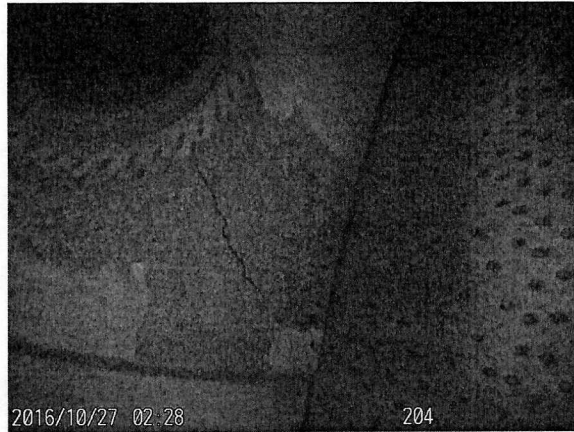
Figure 6 Bulkhead Shell for cracking in zone A
