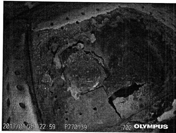
Figure 10 cracking that has led to 1 partially detached stud (OBL1 segment)
