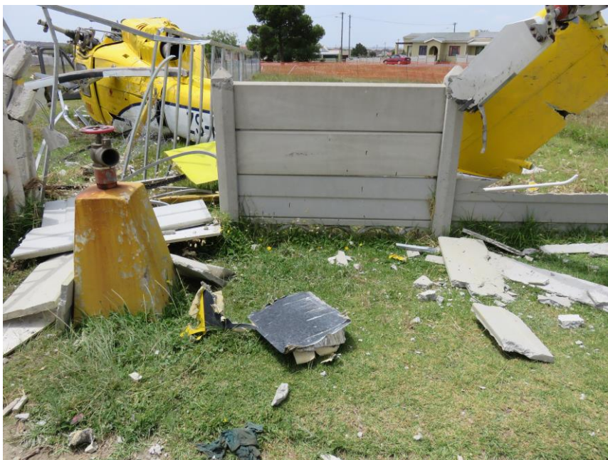
Figure 3: Damage to the concrete perimeter fence, wire fence and gate.
