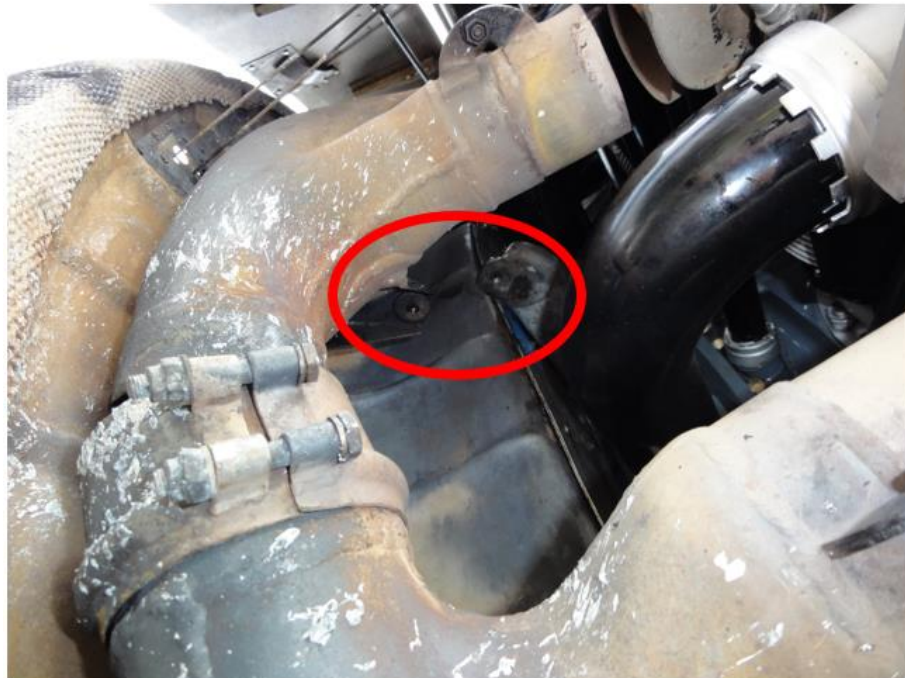
Figure 6. One of the three fittings where the screw joints were missing between the exhaust collector and the engine.
