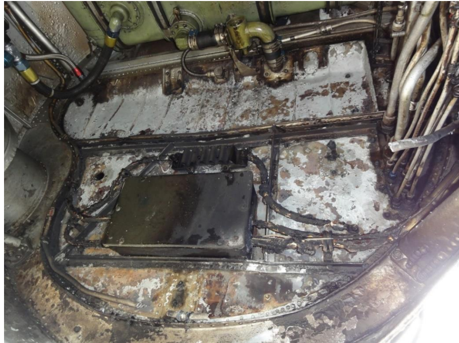
Figure 9. Fire damage in zone 3. Cables on the firewall to the accessory compartment have melted and burned.
