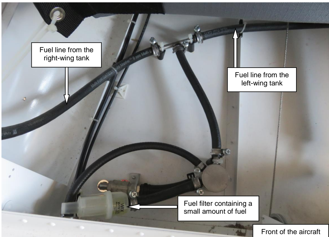
Figure 4: Fuel lines from the left- and right-wing tanks feeding under gravity into a T-fitting (this fuel plumbing is installed behind the two seats)
