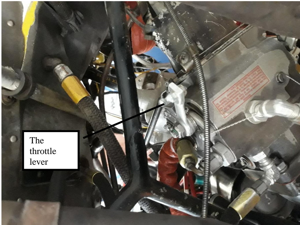
Figure 7: The number 2 engine throttle lever which is missing a throttle control cable end fitting.
