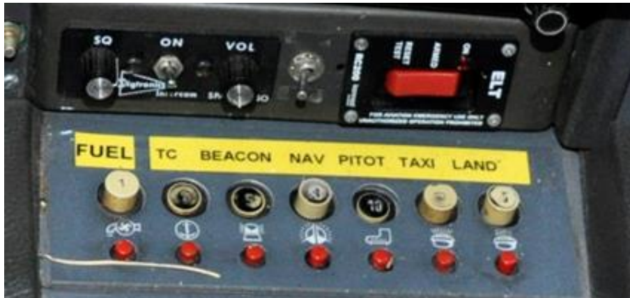
Figure 23. The electrical panel for switches on SE-MKV at the time of the accident. Note that switches for memory items are turned off (pushed out position).
