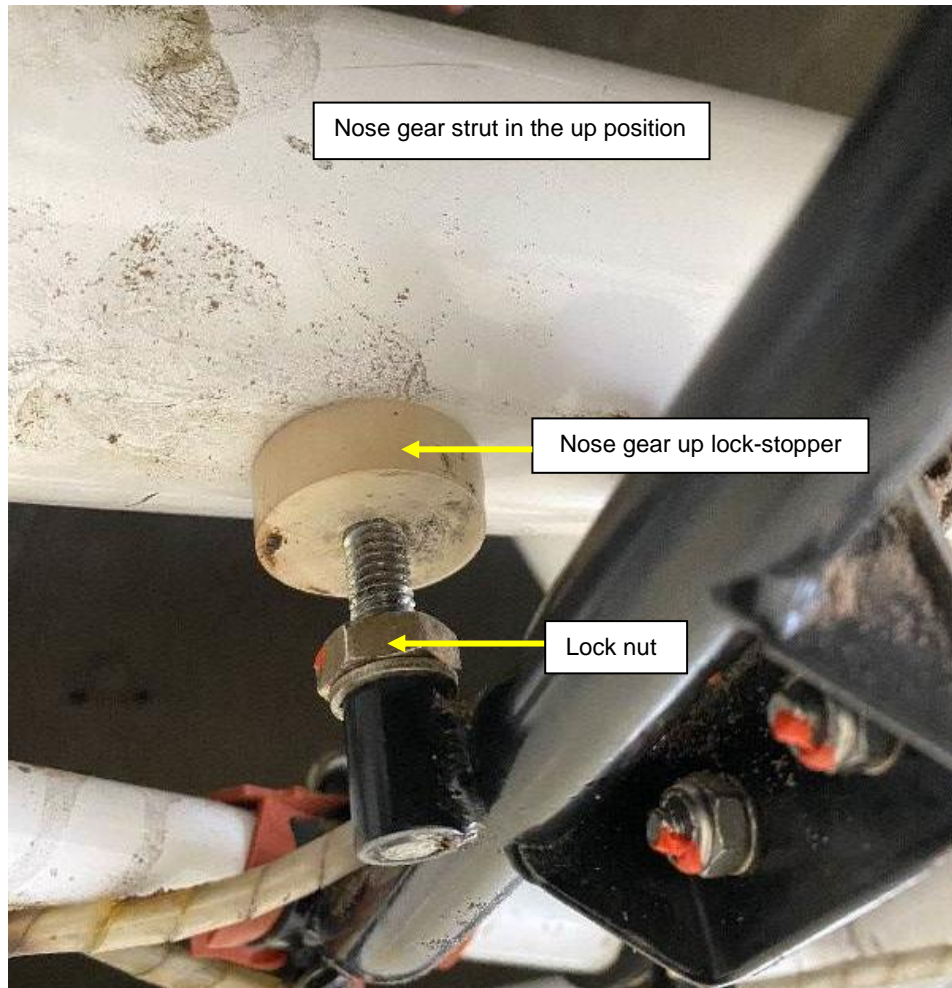
Figure 10: Nose gear up lock-stopper and the lock nut (nose gear in the up position).
