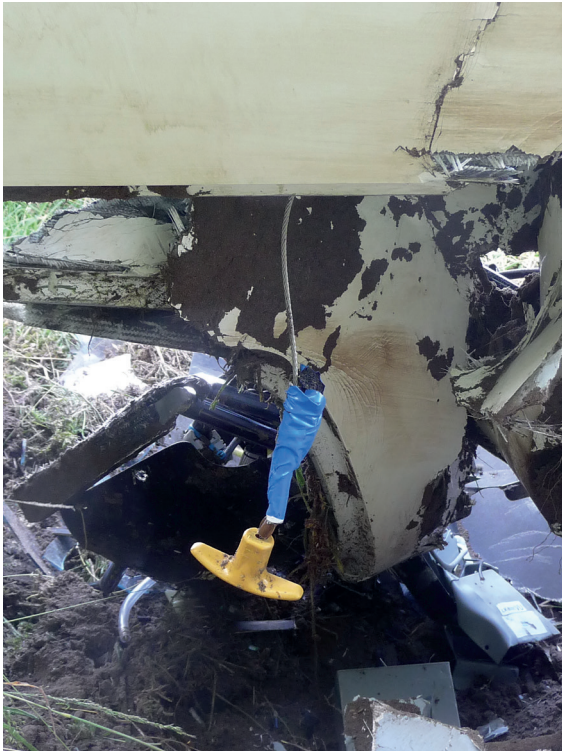
Figure 6: The temporary repair of the molded sleeve, as found at the accident site. (Source: Dutch Safety Board)
