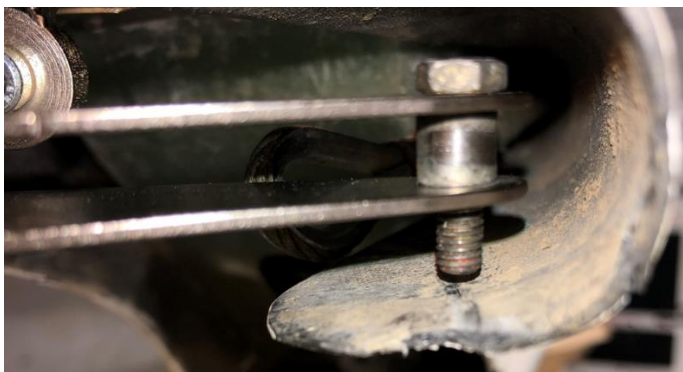
Figure 10. The M8 bolt loosened one and a half turns with a new attachment and rudder yoke mounted.
