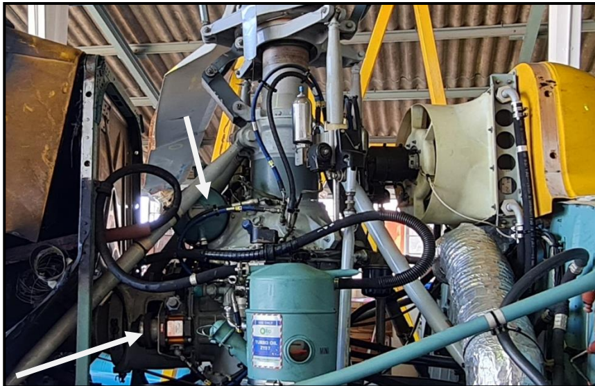
Figure 5: Hydraulic reservoir and pump found intact post-accident.
