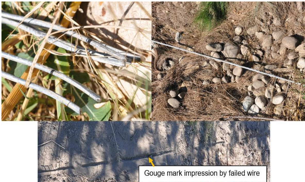
Figure 2: Top-left image: The failed earth conductor. Top-right image: The earth conductor found near the trees. Bottom image: The gouge mark made by the earth conductor.
