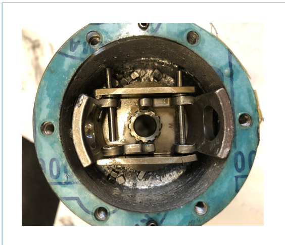
Figure 11: Debris found inside the governor housing. (Source: Dutch Safety Board)
